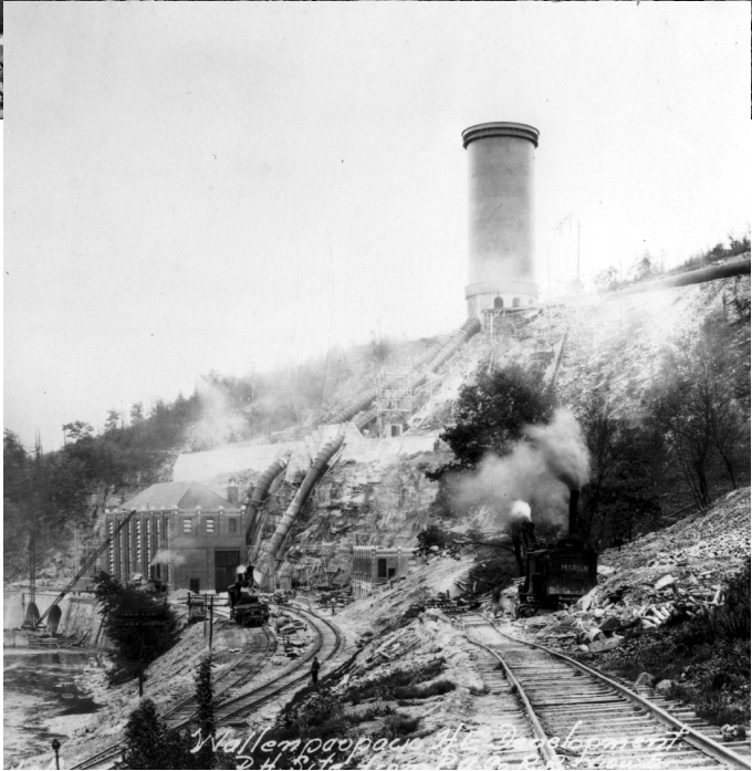
While the dam was under construction three-and-a-half miles away, the seldom-seen Wallenpaupack Hydroelectric Station and its tall surge tank were taking shape down at Kimbles, Pa. Smoke from many steam engines obscures detail in the center of the photo.
